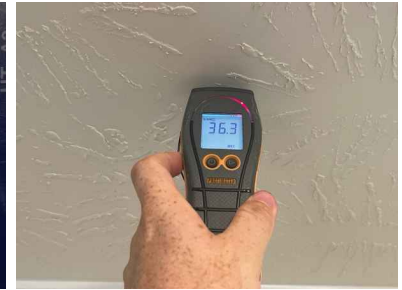
Dining Room confirmed wet
