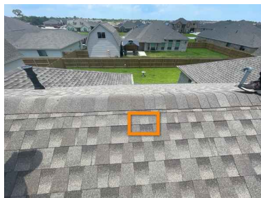
Improper nail location detail
